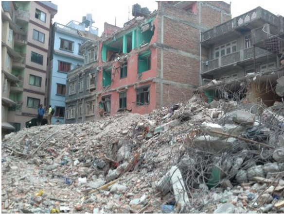
Figure 4. Severe damages to the building in Kathmandu.
